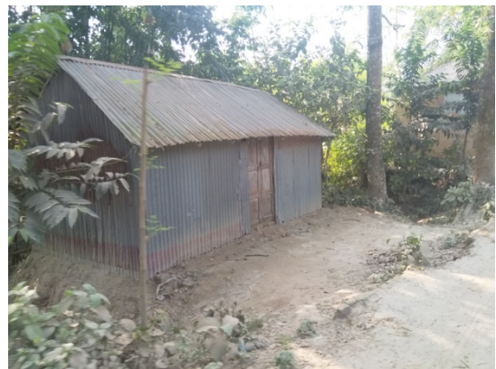
Embankment side settlement
