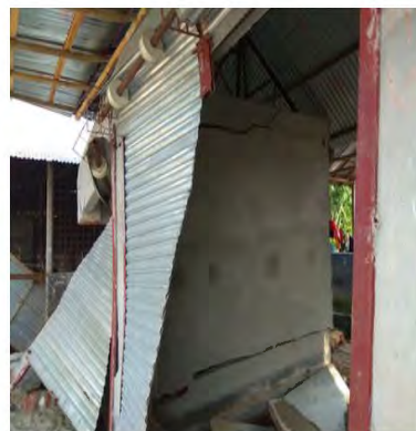
6. n) Erosion affected business shop
