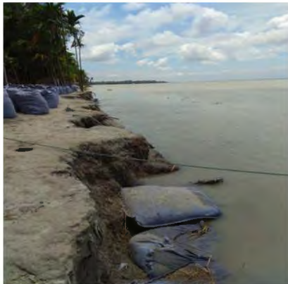
2. a) Bank erosion
