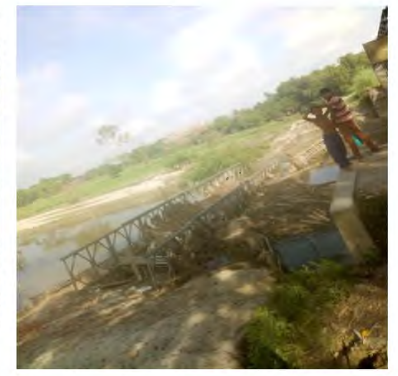
6. l) Collapsed bridge
