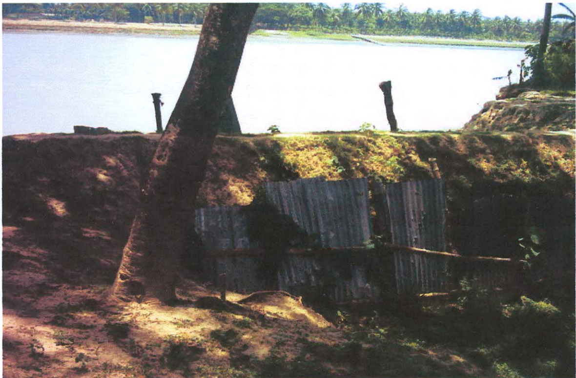
Plate 4: Damage point by cutting embankment
