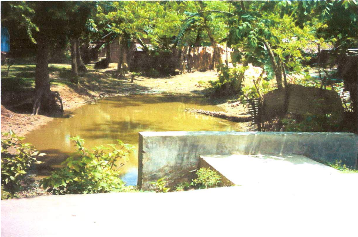
Plate 5: Canal encroachment by settlement
