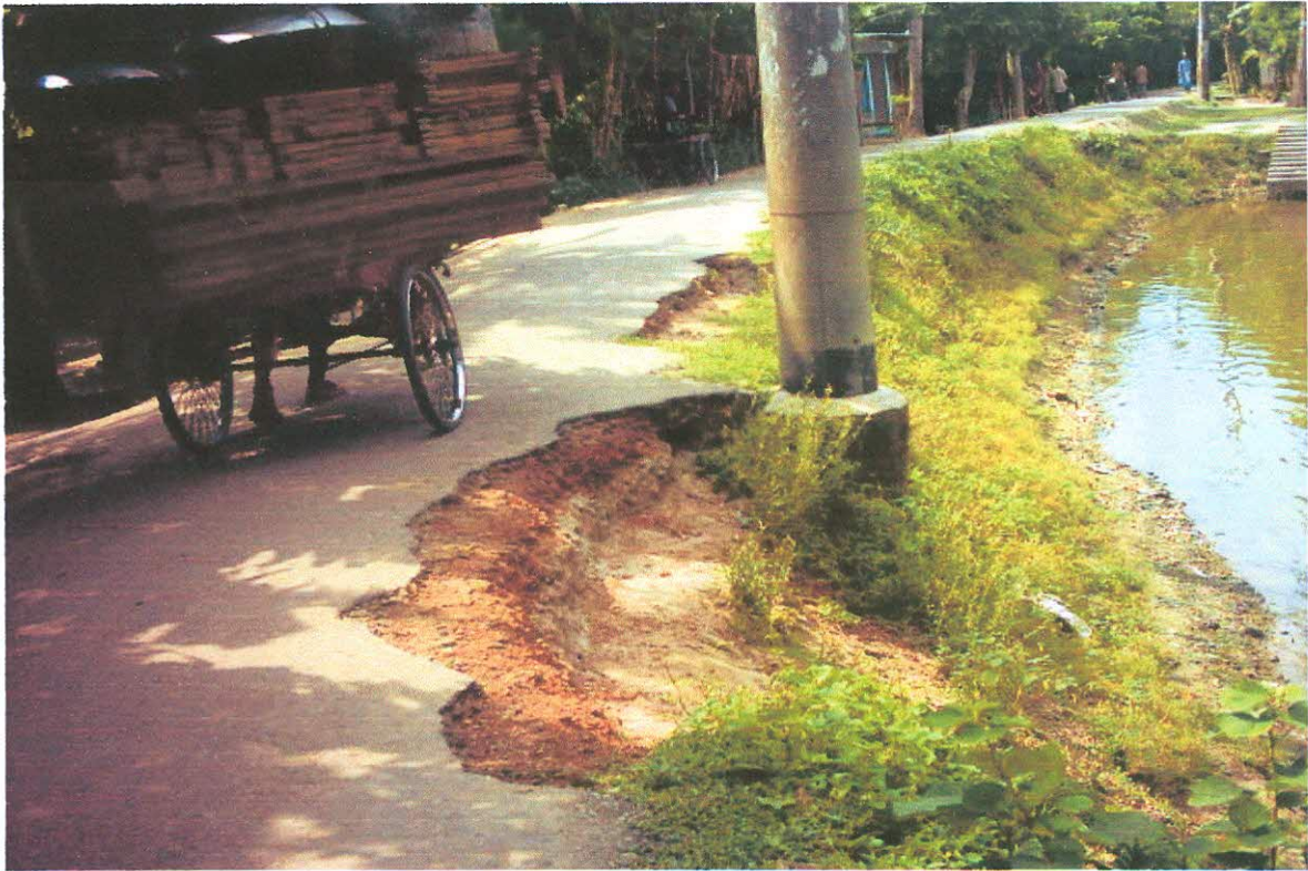
Plate 3: Damage point where major maintenance is required
