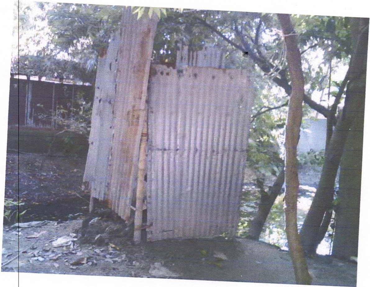
Picture 3: Condition of latrine of an illiterate family of Bangla Bazar village
