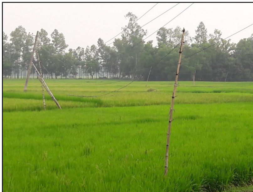
Figure: 6.4: A view of electric wire was pulled by bamboo in the study area.
