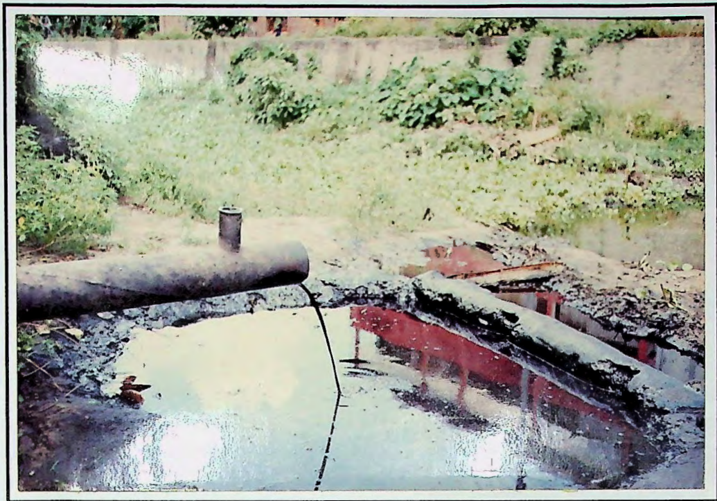
Photograph 12- Discharge pipe showing release of power house effluent (spot-2).
