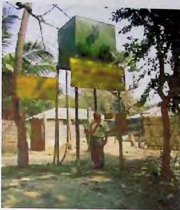
Fig.- 3.5 : Water tank from which gravity feeds the houses.
